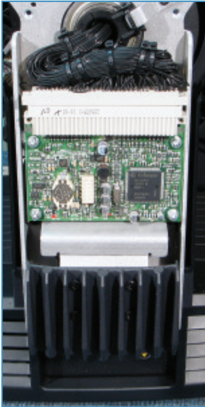
Figure 17 - Main control electronics
